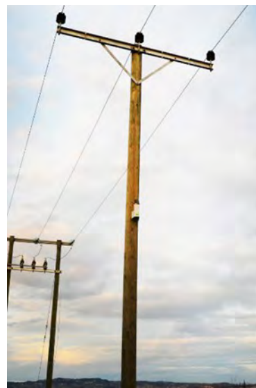
Pole Mounted Indicator
